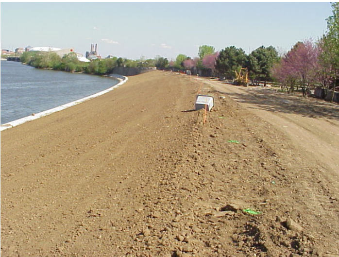
Prepared installation site that is free of weed, clods, stones, roots, sticks, rivulets and gullies.
